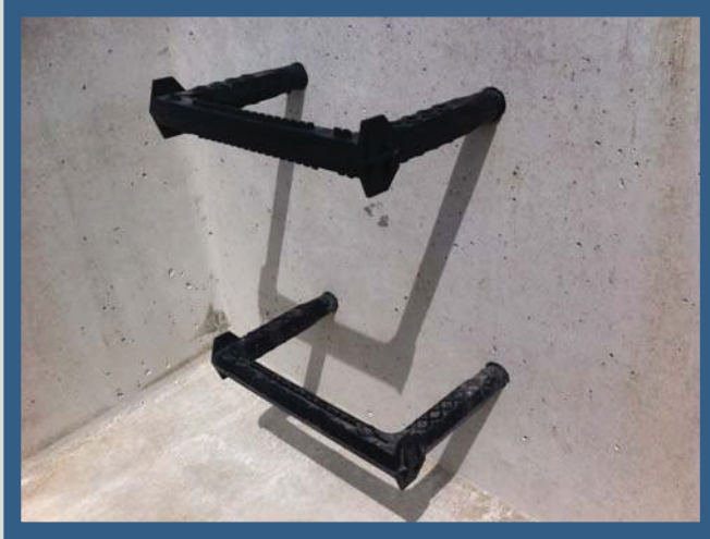
Manhole Ladder Steps
